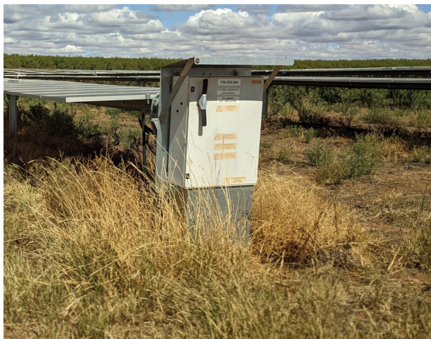
Unmanaged vegetation at string commander box.
